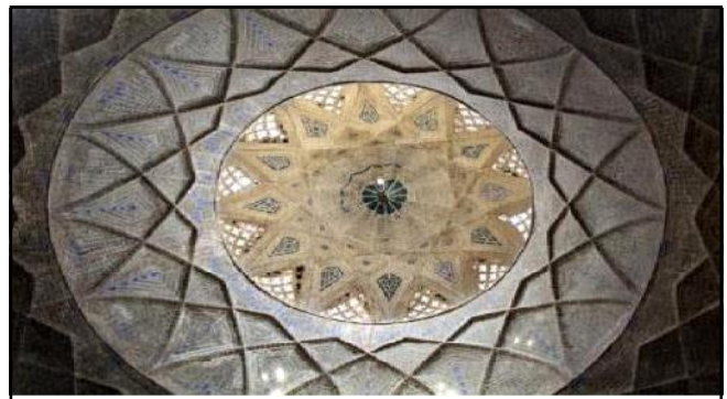
Fig. 7 : D2, Kar-bandi, bazar khan, Yazd, Iran, becoming one of decorative and structural roles
