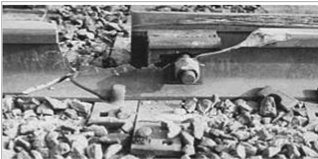
Fig. G : Fracture in rail due to bolt-hole crack
