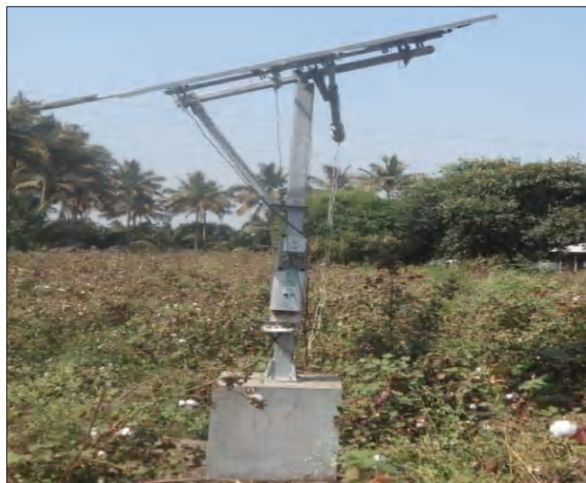
Fig A: Side view of installed solar PV system
