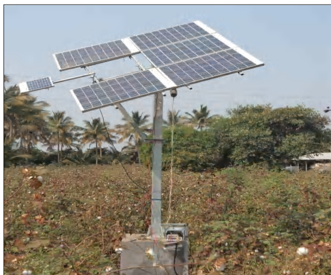
Fig B: Designed solar PV system installed at site
